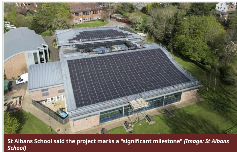
Figure 2: The School's new 185 kW solar installation, completed June 2026. Image: St Albans School, via the Herts Advertiser.
